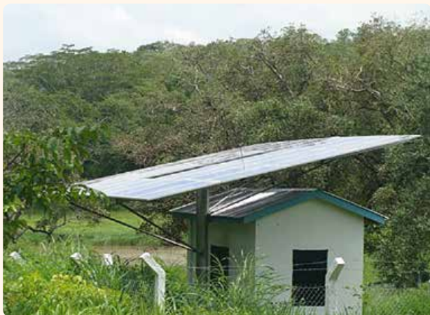
A 6.12 kW Solar Water Pumping System at Misufini Village, Mtwara (R)
